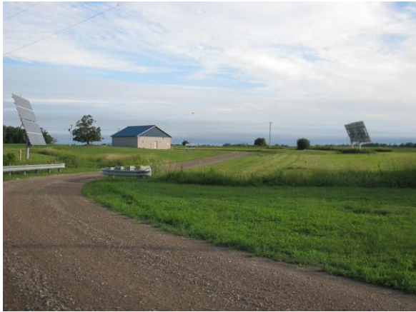
10 kw Solar Trackers at Seaforth Water Plant
