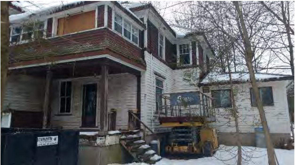
Figure 7: Photo from Centre Street showing the porch to be removed for the proposed addition on the north side
