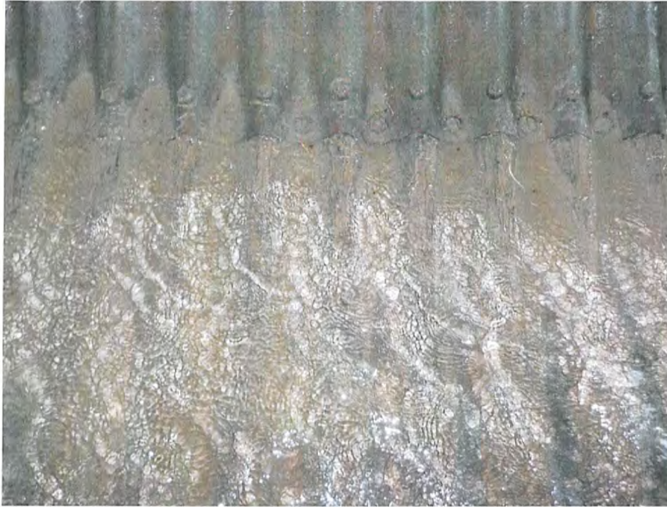
T26 – Bottom Plate Corrosion
